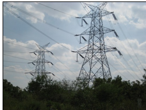
400kV Transmission Line constructed by the Project
