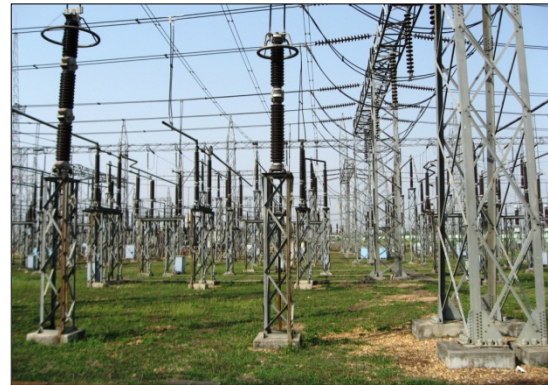
Overview of Equipment at Arambag 400 kV Substation
