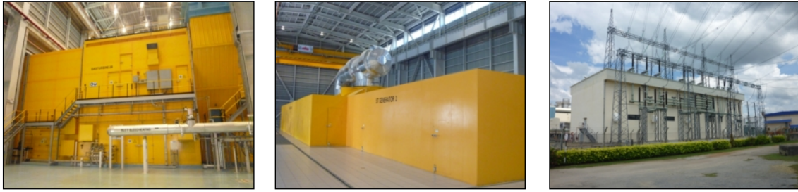
Photo 2: From the left, gas turbine, steam turbine generator and transmission facilities
