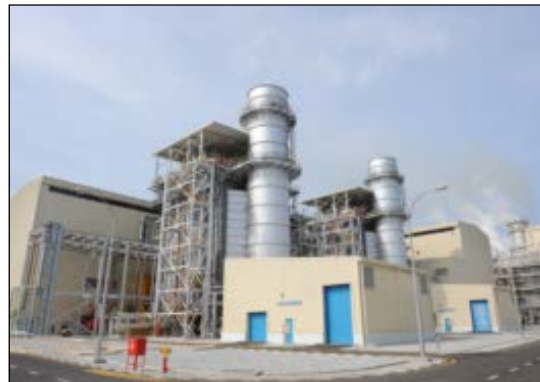
TNB Port Dickson Power Station (Project target power plant)
