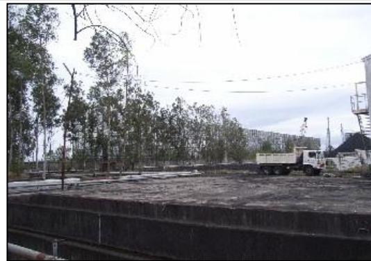
Windbreak Fence installed in the Project
