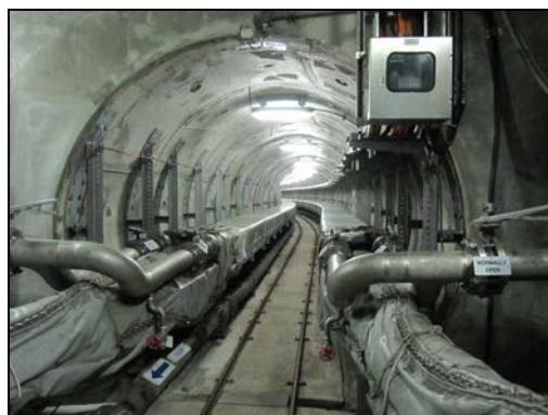
Tunnel and underground cable constructed by this project
