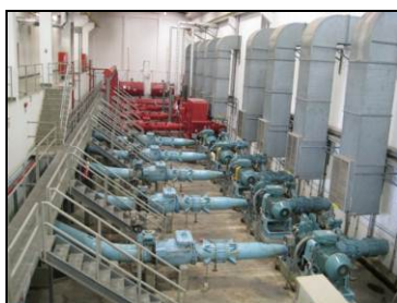
Water Supply Pumping Station
