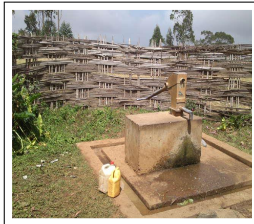
A water facility provided by the project
