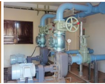
Distribution pump (Nhon Hoa)
