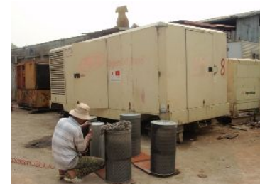
The air compressor on regular maintenance at CCTT
