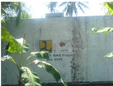
Water Reserve Tank
