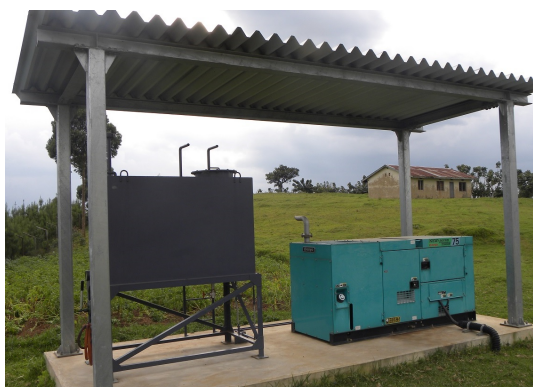
Figure 13: Emergency Generator for Kyeriba MW Transmitting Station (The one on the left is a diesel fuel storage tank.)
