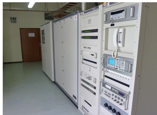
Figure 12: Transmitting Equipment inside Mawagga Transmitting Station
