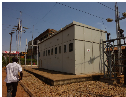
Procured 33kV Switchgear (At Iganga Substation, Iganga District, Eastern Region)
