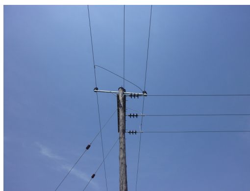
Figure 9: Developed 33kV Distribution Line (Itanda area, Iganga District, Eastern Region)
