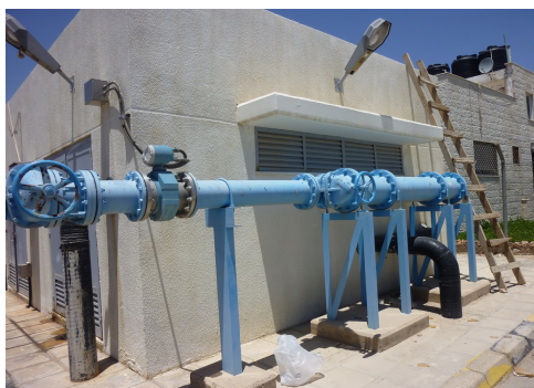
Photo 5: Renewed Pumping Facility (Batrawi Pumping Station)
