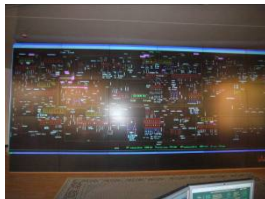
SCADA Video Wall
