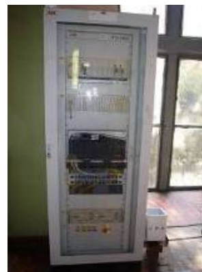
SCADA-related Facility in Yerevan Power Plant
