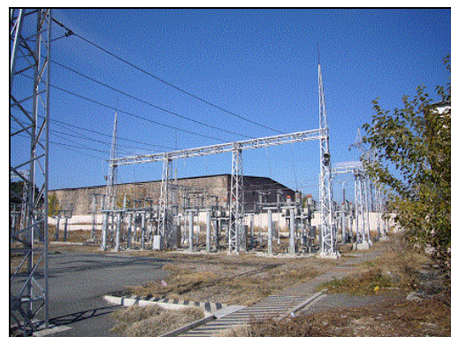
Rehabilitated Echmiatsin Substation
