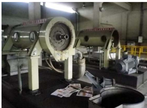
Sludge Centrifugal Dewatering Units (Penha WWTP)
