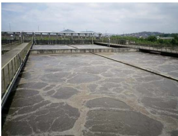
Secondary Treatment Facility (Alegria WWTP)
