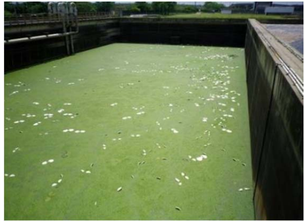
Secondary treatment facility not available for operation (Pavuna WWTP)
