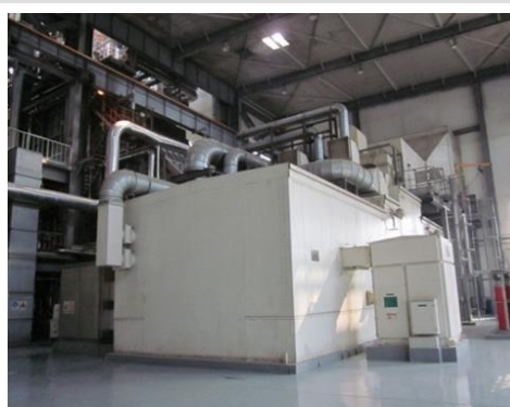
Gas turbine (stored within a soundproof structure)
