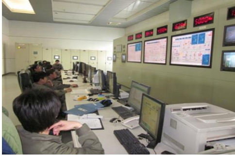
Figure 9 : Automatic control room (decentralized control system 22 )
