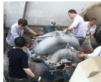
Figure 13 : Inspecting a coolant circulation pump
