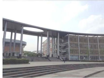
Student Science and Technology Center of SWUST. Located in Mianyang, the city closest to the center of the Great Sichuan Earthquake. All exterior walls fell off in the earthquake, however, they were promptly repaired.
