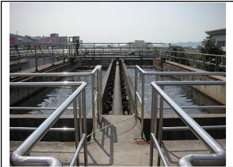
Sedimentation Tank of the Linjiangxi Sewage Treatment Plant
