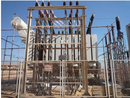
Substation installed by the project
