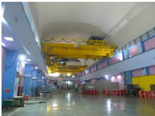
Inside of the power house
