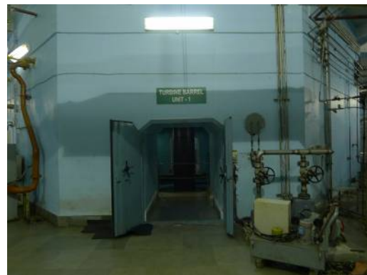
Pump-turbine of Unit 1
