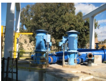
Water Intake Facility
