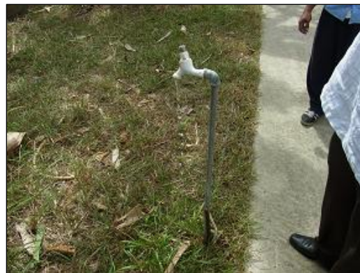
Faucet for Reused Water (Mactan)
