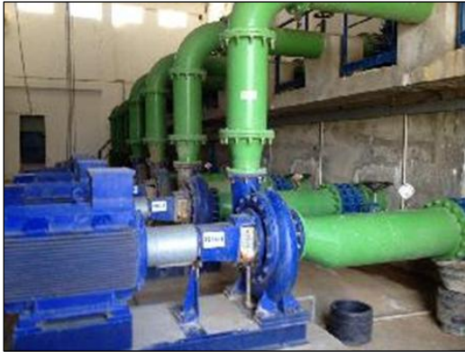
Pumping Station (Fernana)
