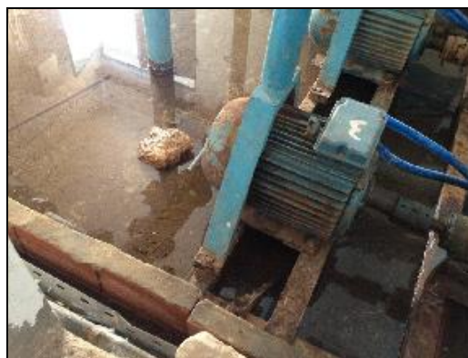
Inundated pumping station (Medenine)
