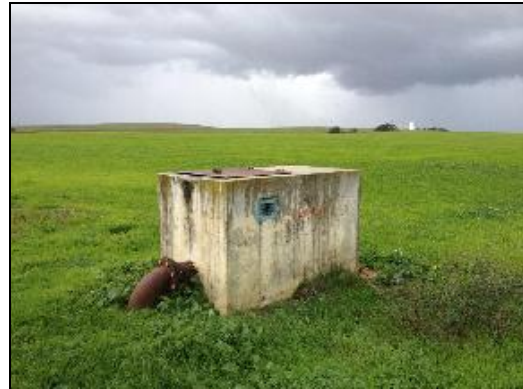
Distribution valve for irrigation
