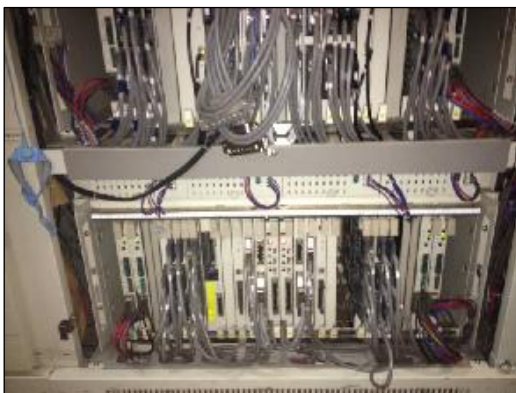
Switchboards: empty slots can be seen
