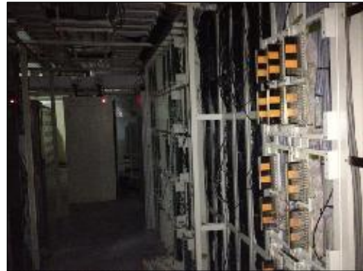
Switching Station (Harare)
