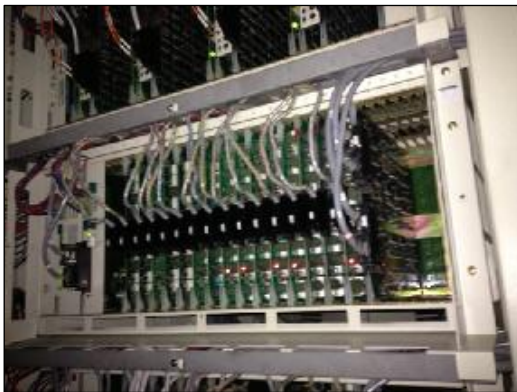
Switching board: empty slots can be seen
