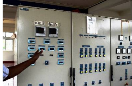
(Upgraded Equipment of Logwood Water Treatment Plant)
