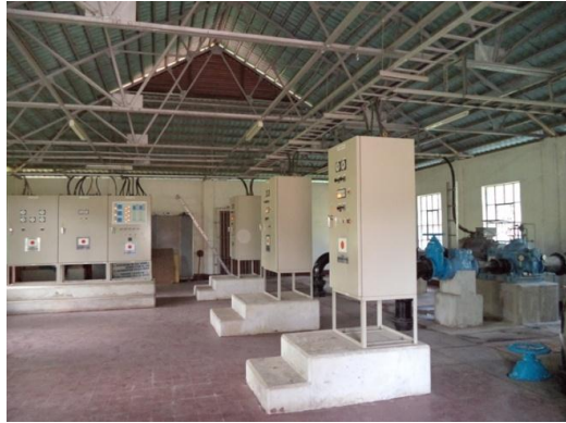
Photo 1: Saateni Station Transmission Pump House
