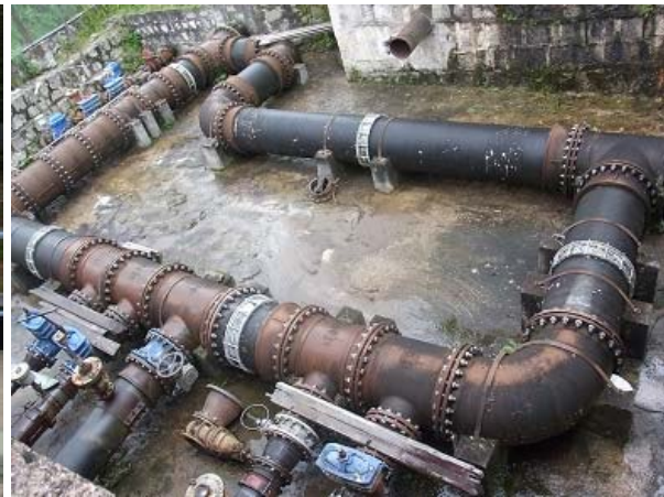
Transmission pipeline leaving from the Picacho WTP
