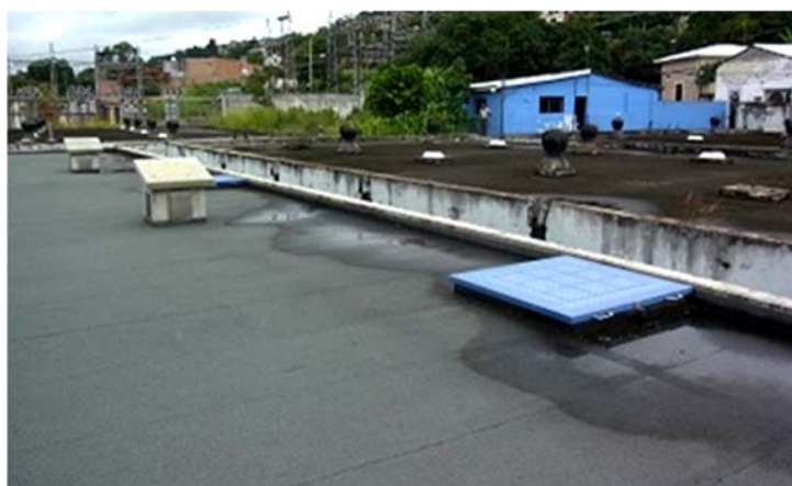
Distribution tank in the La Sosa distribution area
