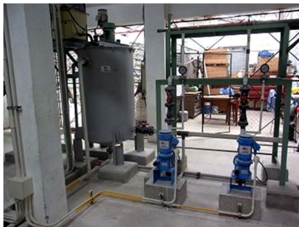
Aluminium solidifier injection device at the Picacho WTP
