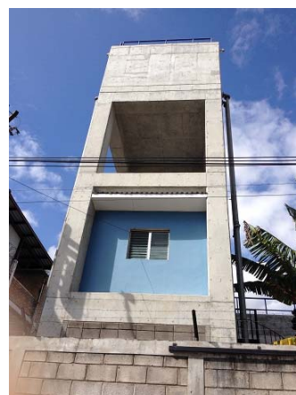
Distribution tank in the San Francisco distribution area
