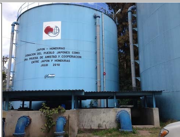
Distribution reservoir at the Olimpo 1 Water Distribution Center
