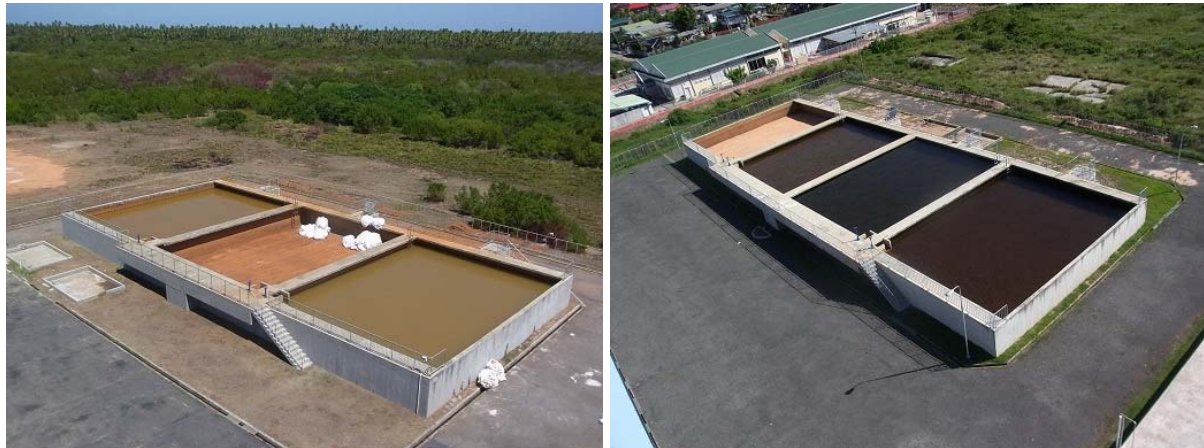
Slow sand filter bed at the No. 56 Village WPT (left) and Queenstown WTP (right) 17
