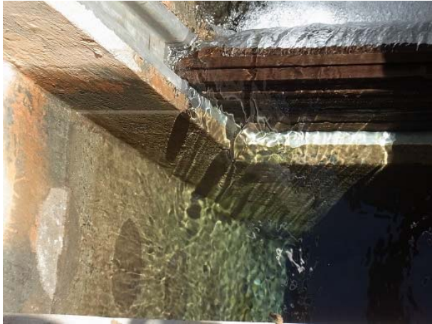
Purified water (No. 56 Village WTP)
