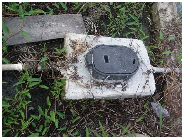
Installed water meter
