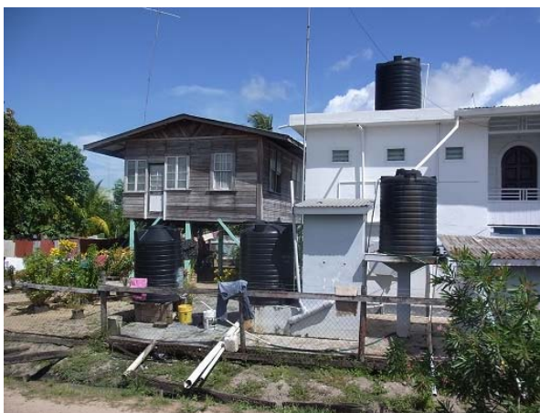
Water tanks installed at ordinary households
