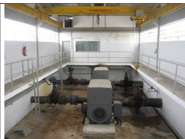
Figure 7: A Pump Station for the Semi-Arid Water Conveyance System
