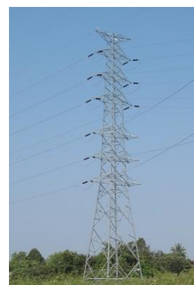
Photo 2: A transmission line tower for 4 circuits (Near Pakxan substation)
