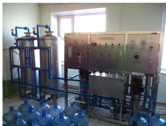
Water purifier purchased with the sub-loan from this project (Purified water manufacturer in the suburb of Ulaanbaatar)
