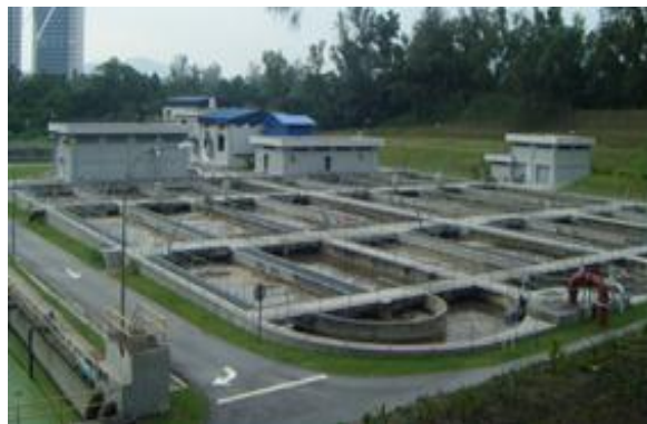
Damansara Sewerage Treatment Plant
