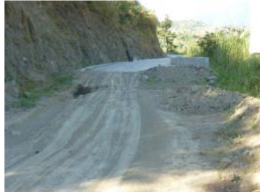
Photo 2: (3-b) Unpaved section of Cervantes-Sabangan Road
