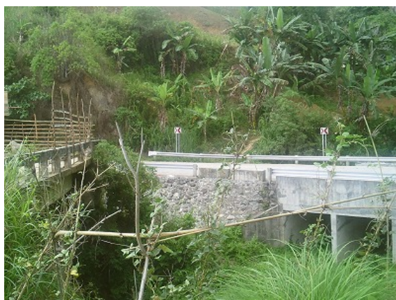
An old bridge on the left was abolished and the roads were rerouted with installment of a new box culvert (Section 2)
