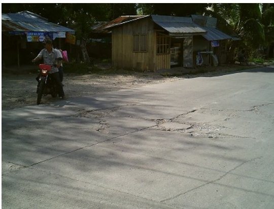
Damage on the Road Surface (Section 1)
