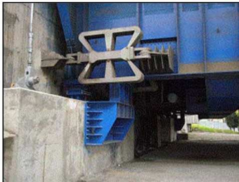
Dampers 5 installed at Golden Horn Bridge
