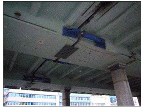
Damper installed at Mecidiyekoy Viaduct
