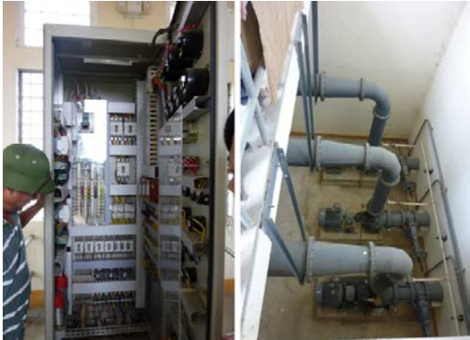
Photo 2: Control Panel (left) and Pump Unit (right) inside Nam Trung Pumping Station
