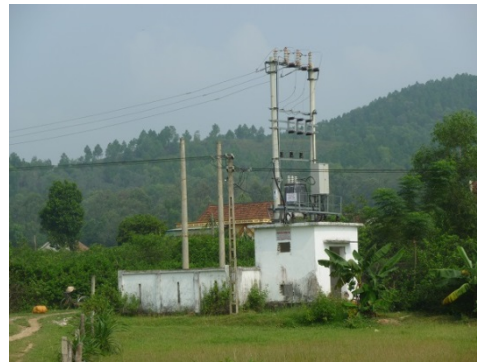
Photo 4: Rehabilitated electric power substation
