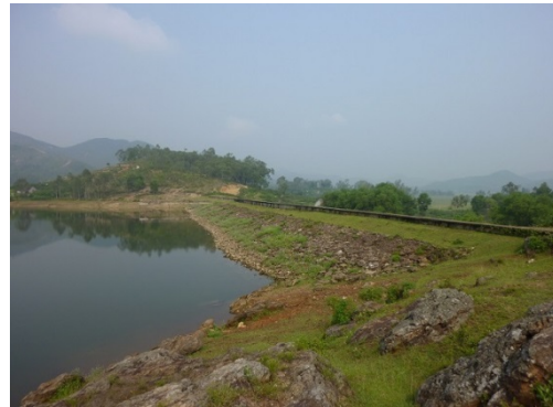
Photo 6: Ho Thanh reservoir (countermeasure to reservoir leakage was taken from the center to the right-hand side of the photo)
