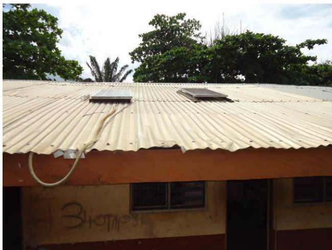
Solar panel installed in a school at Akyerekrekrom
