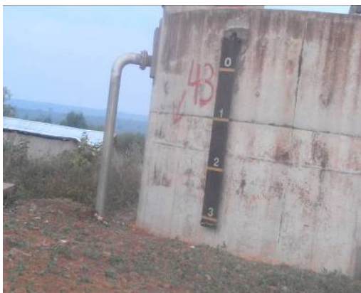
A full water tank in Rwamagana district
