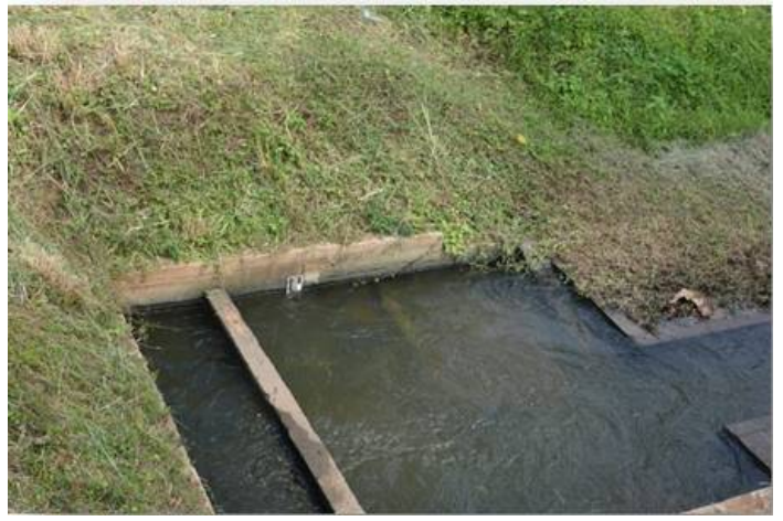
Constructed water controller and canals in model site
