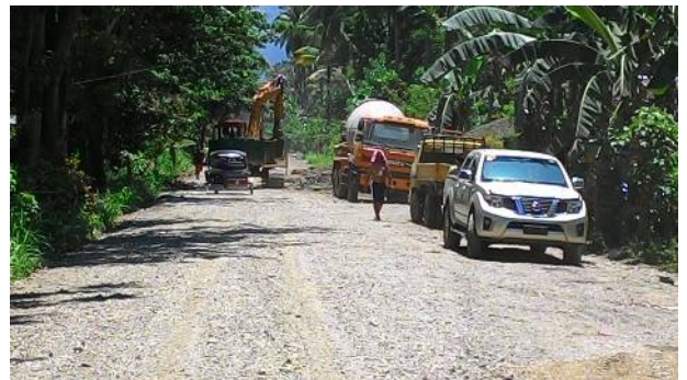
(Construction of access road to Maruyog Resort: The necessity of road was verified by the data collected by the Tourism Data Management System which shows an increase in the number of visitor arrivals in the municipality of Brooke's Point.)
