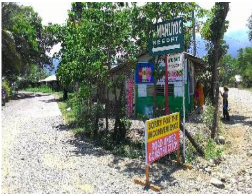
(Construction of access road to Maruyog Resort in the municipality of Brooke's Point, Palawan province. The project was proposed by the Municipal Tourism Office and was approved and funded under DOT-DPWH Convergence Program.)
