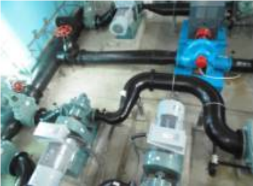
Pump house and pipes of a transmission pump
