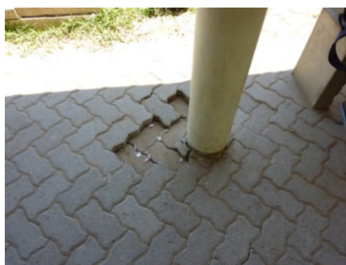
Photo 12: Subsided blocks (Nkobe school)
