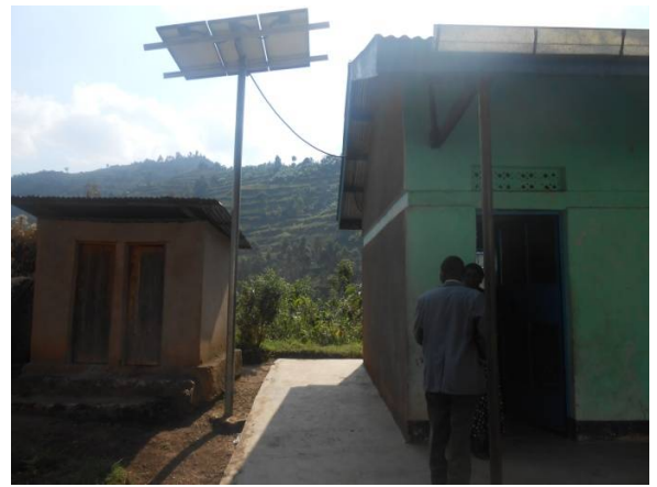
Solar Panel for the Freezer
