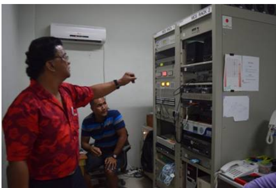
Technician room and equipment provided by the project
