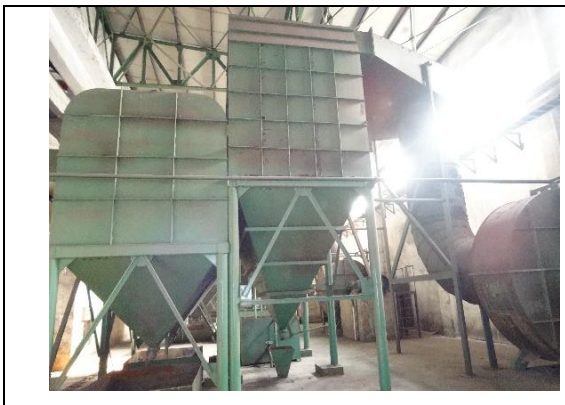
Photo 2: A 40 t Boiler Installed in a Boiler House in “Gaoxin District”
