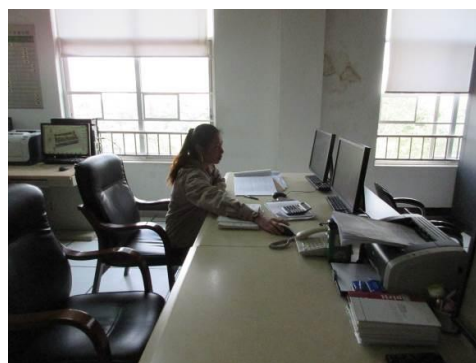
Photo 5: The central control room of the Treatment Plant
