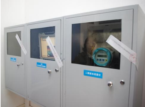
Photo 6: Treated water monitors
