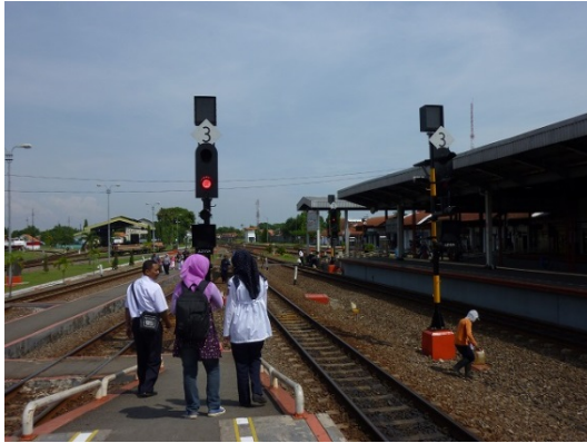
Photo 7: Installed Signal Equipment
