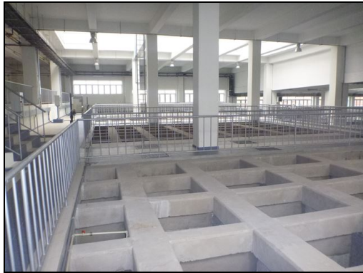
Photo 1: Inside of Water Treatment Plant
