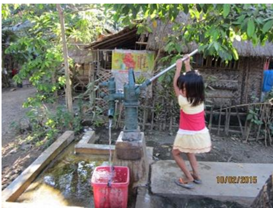
Water supply facility of this project Calintaan, Occidental Mindoro
